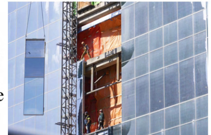
Building retrofits are critical for the energy transition. CHRISTINE WISCH / ISTOCK / GETTY IMAGES
